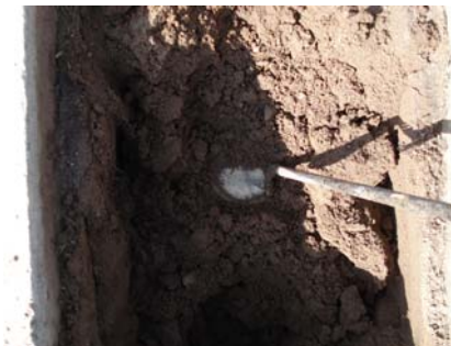
Meter covered with dirt
